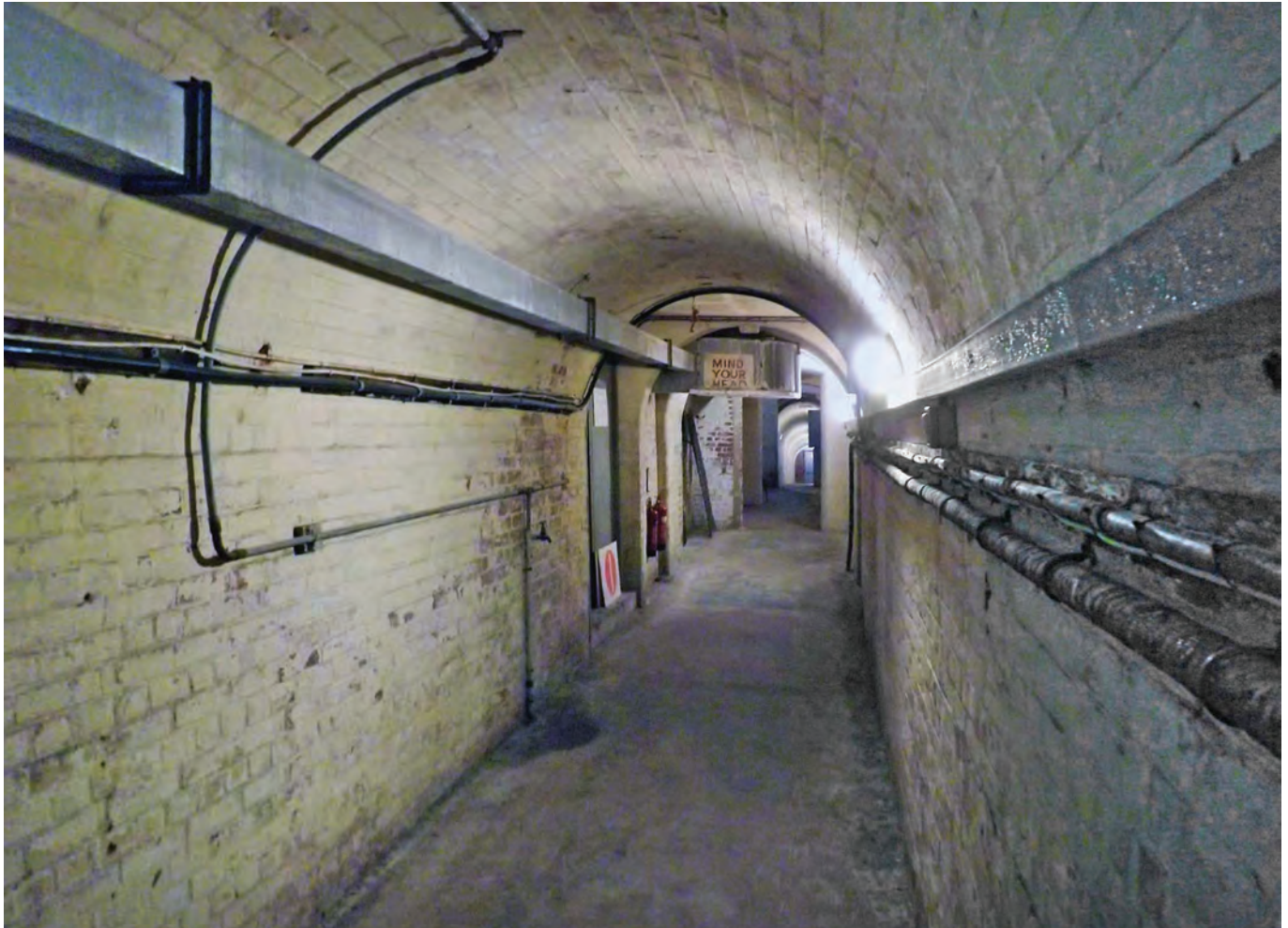
The tunnel to the emergency control centre from the main fort at Widley
